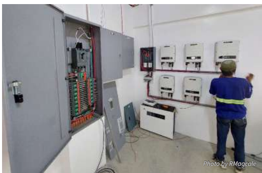
Inspection at the Solar Power System for synchronization to grid
